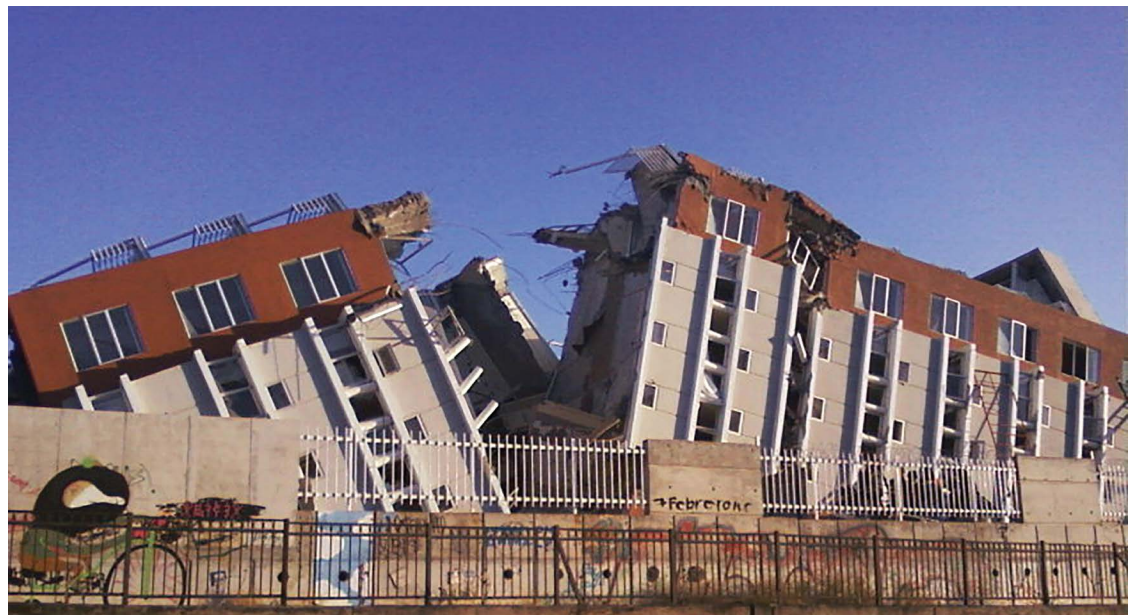
Fig. 1. Alto Río building after earthquake 27F, Concepción, Chile, 2010. (© and Photo: Juan Carlos Briede)
